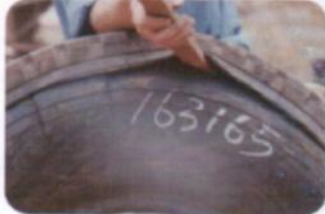
Punctuation and Delaminating
